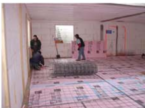
Radiant in-floor heat installed by Johnson Plumbing and Heating
